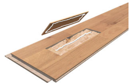
Select and fit a replacement strip. Fill the cavity with polyester filler and press the strip down.
